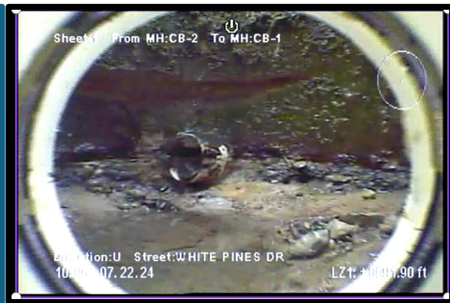
Photo 2 – Storm Drain Filled w/Sediment
